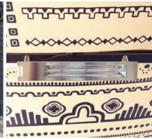
ROOFTOP WITH CEILING MOUNTED SLIMLINE HEATERS
